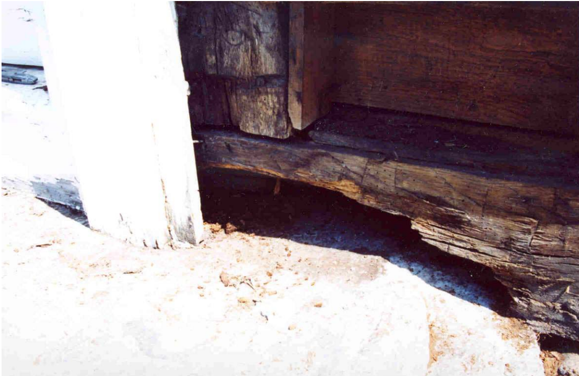
Figure 1. View of sill at west elevation showing area of deterioration where the sill rests on the stone step. Exterior trim removed to expose sill.
