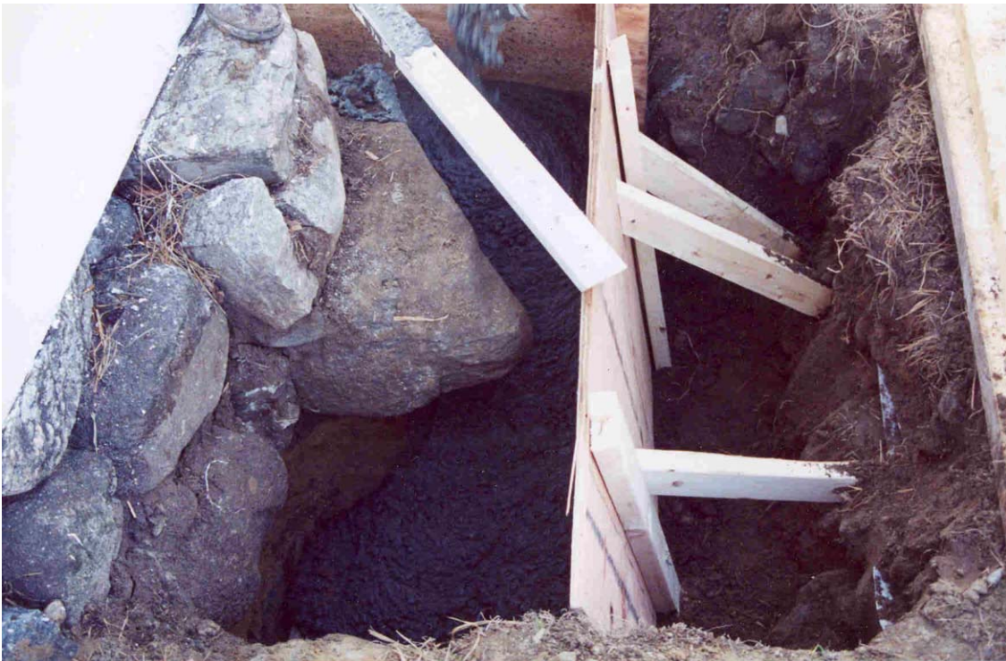
Figure 6. Northwest corner of building showing concrete formwork prior to placement of concrete footing.
