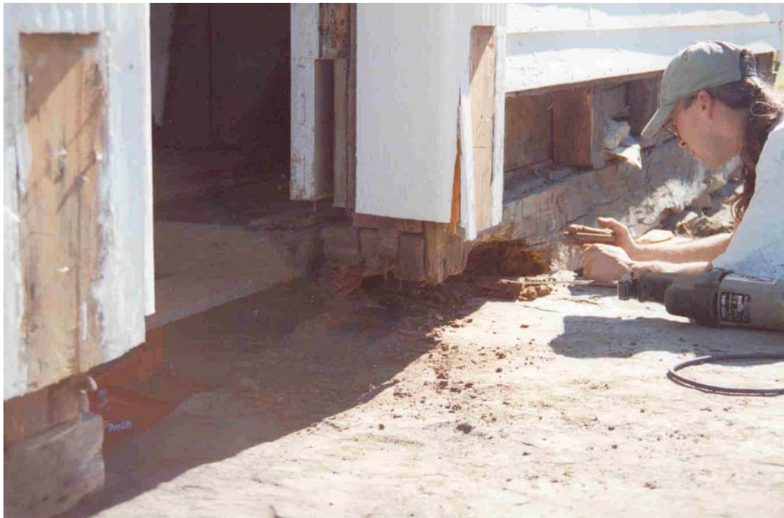
Figure 2. Deteriorated section of sill removed below west elevation door. Note post tenon at right.
