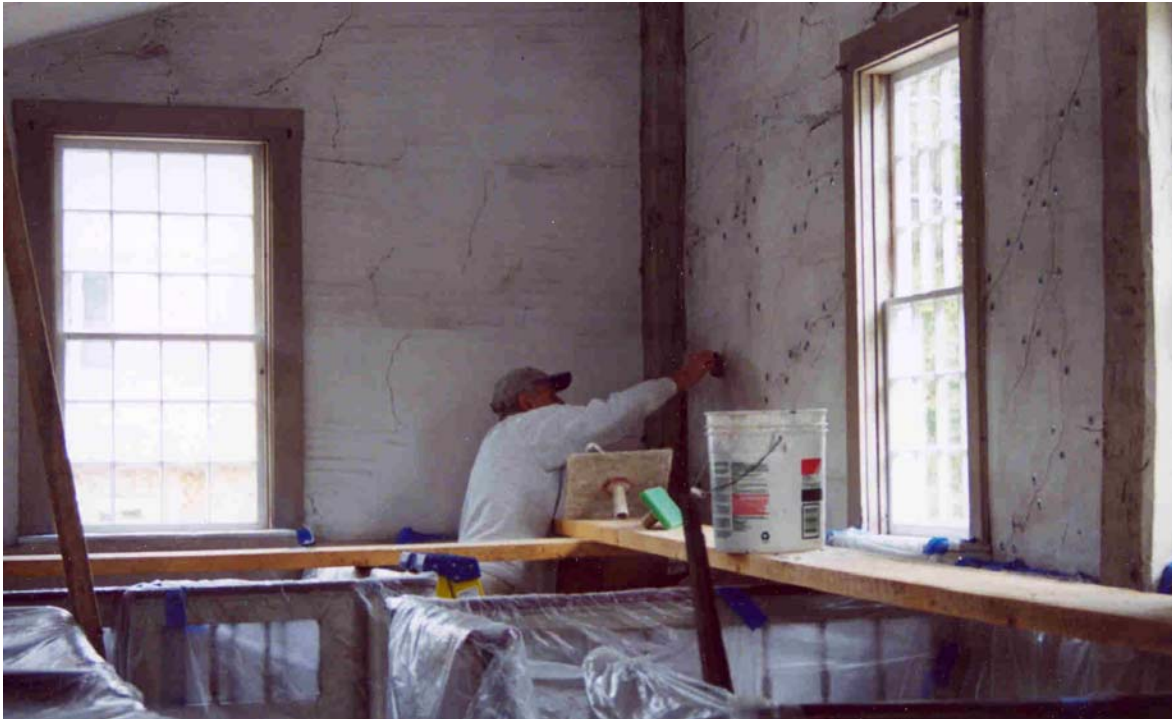
Figure 16.. Filling stabilized cracks in plaster. Note plaster washers along lines of stabilized cracks.
