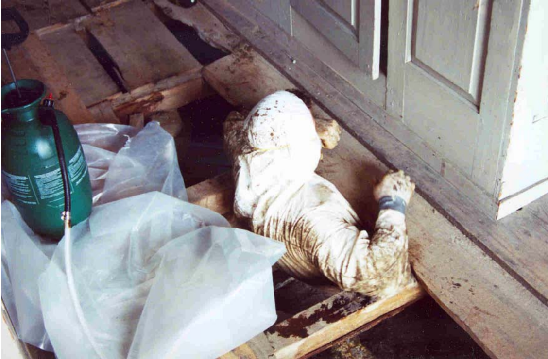
Figure 9. Worker accessing subfloor crawl space. The existing floor framing was found to be in remarkable sound condition.
